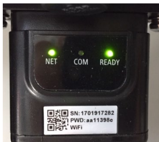
Figure 71 - Irregular communication status between the inverter and adapter
