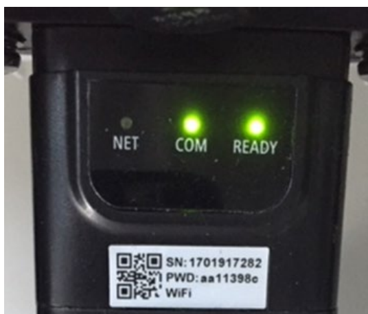
Figure 72 - Irregular communication status between the adapter and remote server
