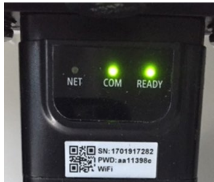
Figure 78 - Irregular communication status between the adapter and remote server
