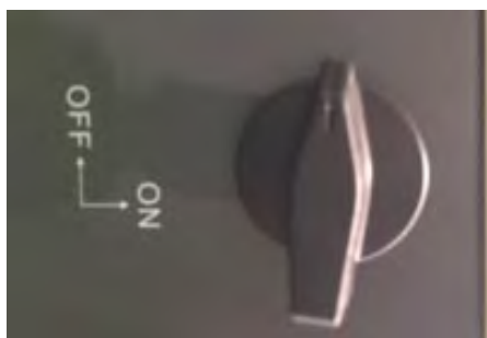
Figure 56 - Photovoltaic disconnecting switch
