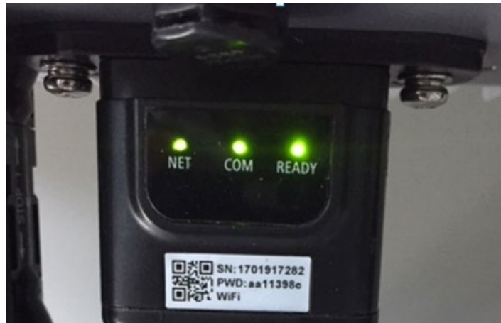
Figure 133 - Final status of LEDs
