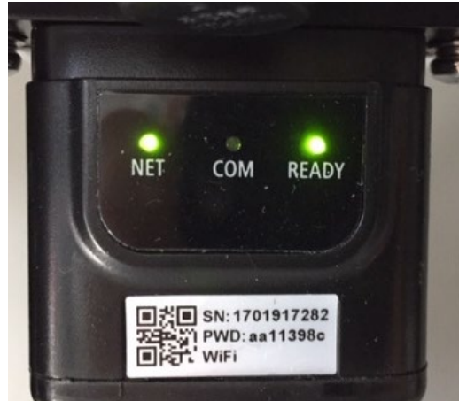
Figure 134 - Irregular communication status between inverter and adapter
