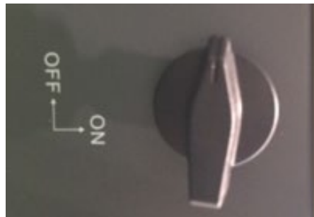
Figure 99 - Photovoltaic disconnecting switch
