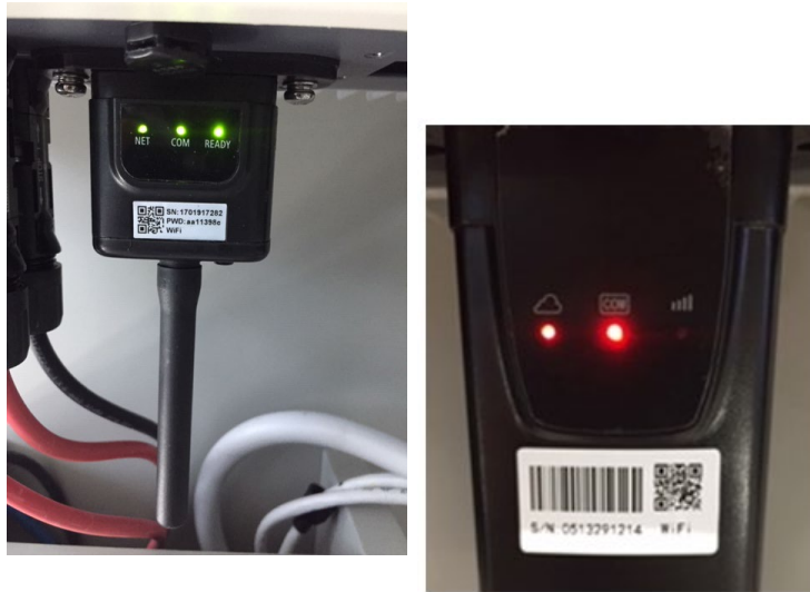
Figure 121 - Final status of LEDs
