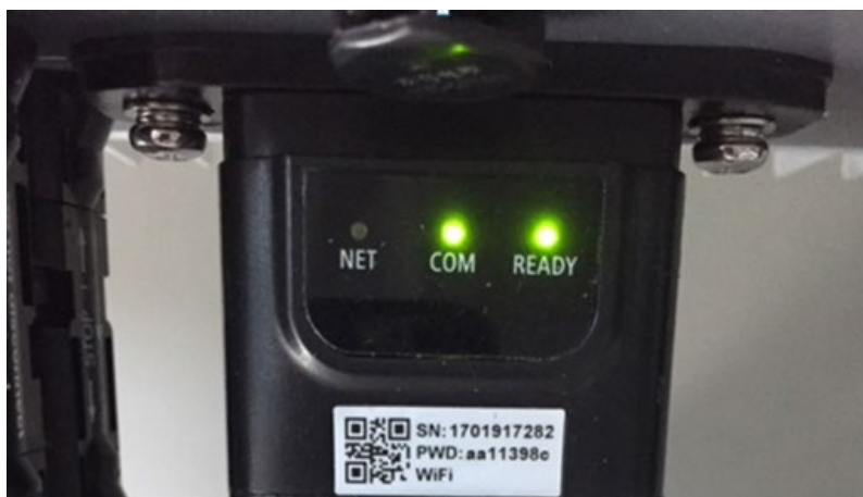
Figure 132 – Initial status of LEDs
