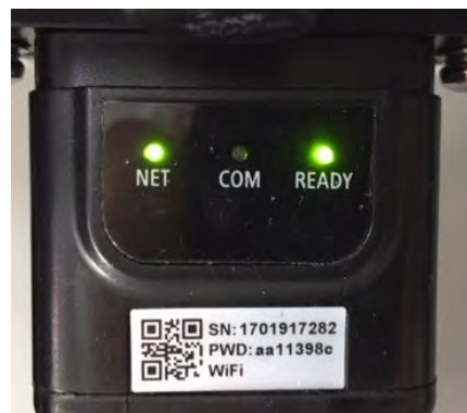
Figure 70 – Irregular communication status between inverter and adapter
