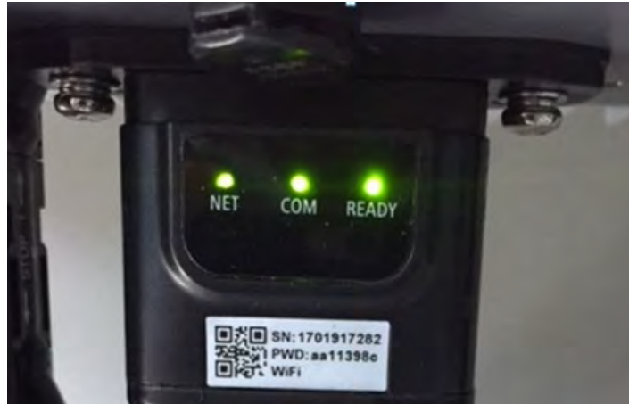
Figure 63 – Final status of LEDs
