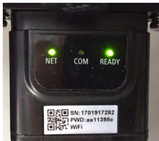
Figure 64 – Irregular communication status between the inverter and adapter
