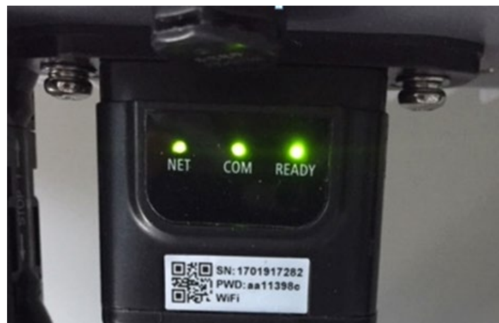
Figure 72 - Final status of LEDs
