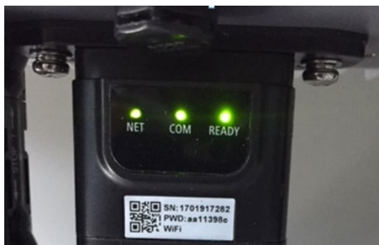
Figure 78 - Final status of LEDs
