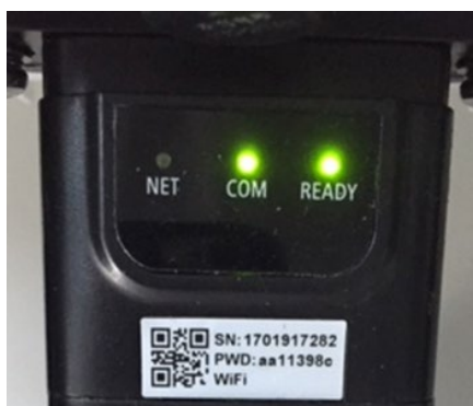
Figure 80 - Irregular communication status between the adapter and remote server
