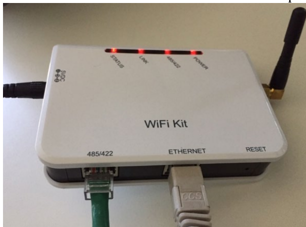
Figure 89 – Ethernet cable connected to the datalogger
