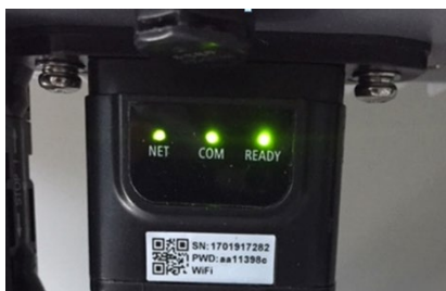
Figure 5-62 - Final status of LEDs
