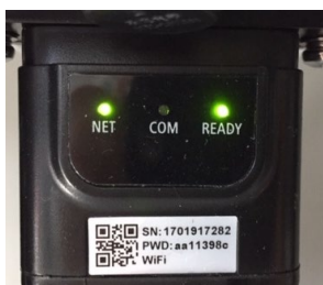
Figure 5-62 - Irregular communication status between inverter and adapter
