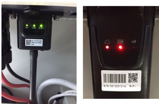
Figure 5-52 - Final status of LEDs
