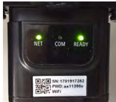
Figure 5-59 - Irregular communication status between the inverter and adapter
