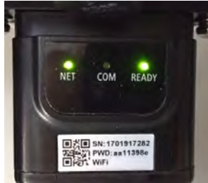
Figure 5-62 - Irregular communication status between inverter and adapter
