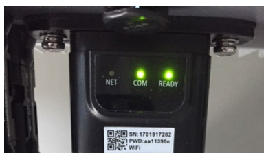
Figure 5-61 - Initial status of LEDs
