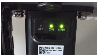
Figure 5-59 - Initial status of LEDs
