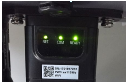
Figure 5-62 - Final status of LEDs
