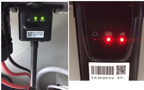
Figure 5-51 - Initial status of LEDs
