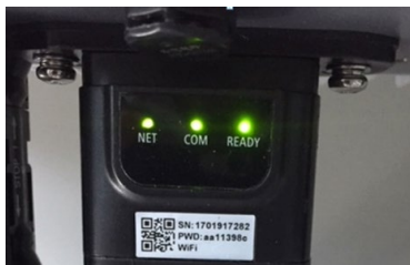
Figure 5-59 - Final status of LEDs
