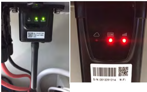
Figure 5-51 - Initial status of LEDs
