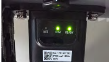
Figure 5-59 - Initial status of LEDs
