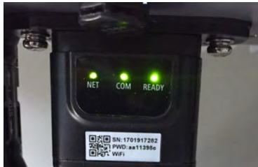
Figure 5-59 - Final status of LEDs
