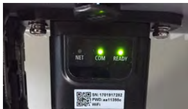
Figure 5-61 - Initial status of LEDs
