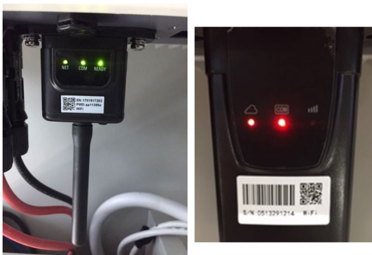
Figure 90 - Final status of LEDs
