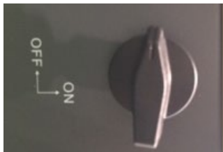
Figure 69 - Photovoltaic disconnecting switch
