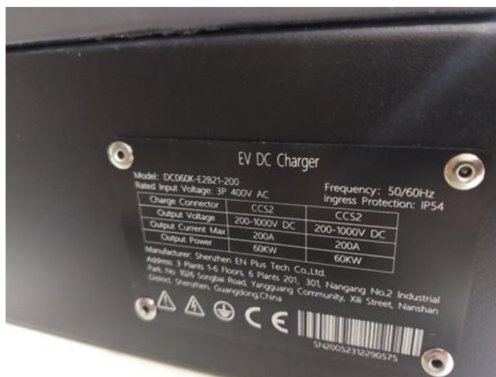
Figure 2 - Labels present on the charging station
